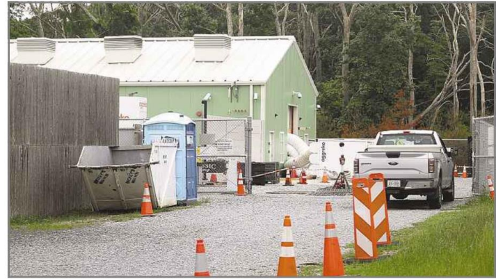
Substation in East Hampton where a fire broke out in May.
